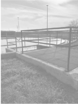
NOTE: REPLACE ANY STEEL SUPPORTS, RAILING AND GRATING AT EFFLUENT BOX WITH ALUMINUM. REPLACE GRATING EMBEDS, SEE DETAIL 1/35-S401
