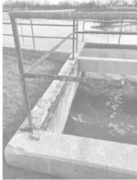
NOTE: REPLACE ANY STEEL SUPPORTS, RAILING AND GRATING AT EFFLUENT BOX WITH ALUMINUM. REPLACE GRATING EMBEDS, SEE DETAIL 1/35-S401
