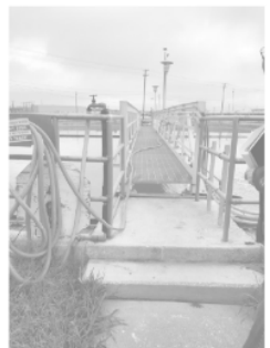
NOTE: REFINISH ALL STEEL BRIDGE ELEMENTS WITH: NEAR WHITE BLAST CLEANING, 1 COAT EPOXY PRIMER 2.5 MDFT, 1 COAT POLYURETHANE ENAMEL 3.0 MDFT
