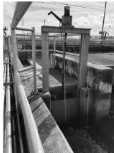
4 40-M141 VIEW OF EXISTING GATE TO BE REPLACED LOOKING SOUTHWEST SCALE: NONE
